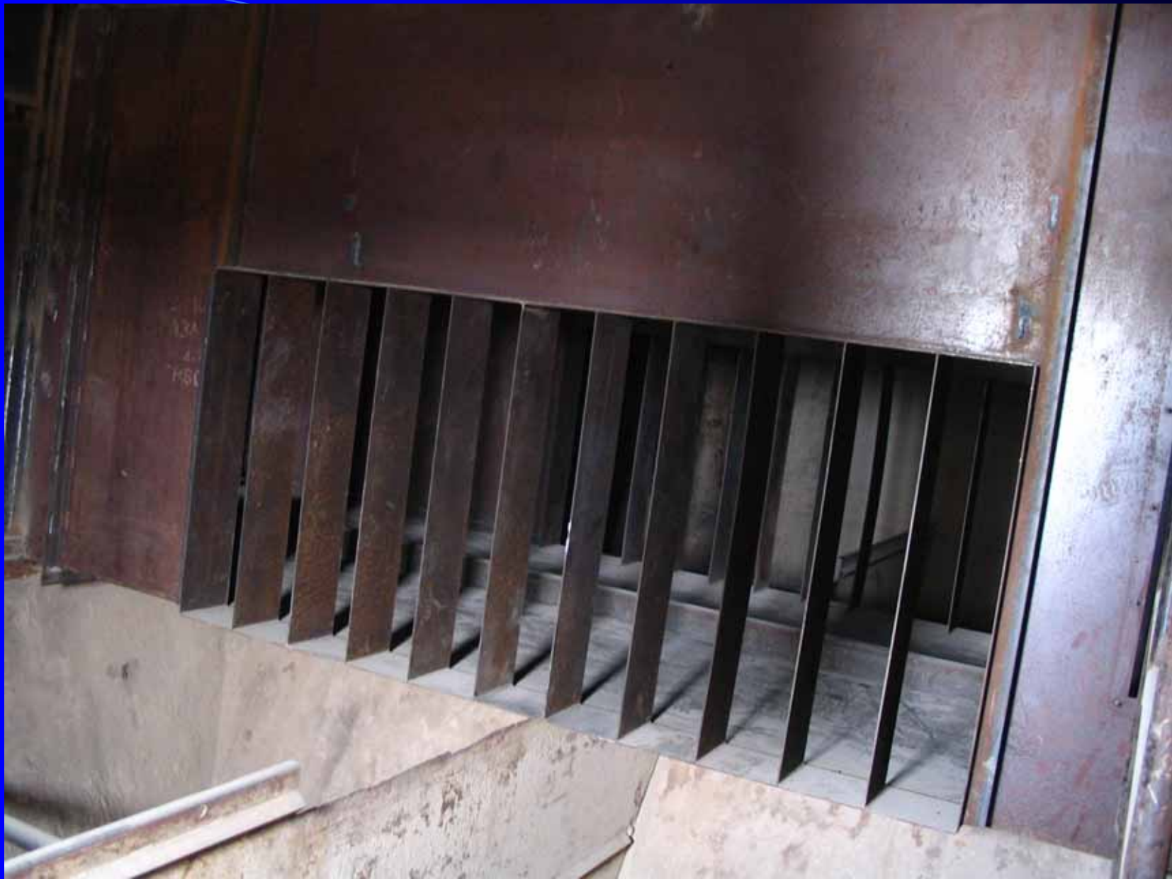
Inlet Plenum Vaned Compartment Entrance
