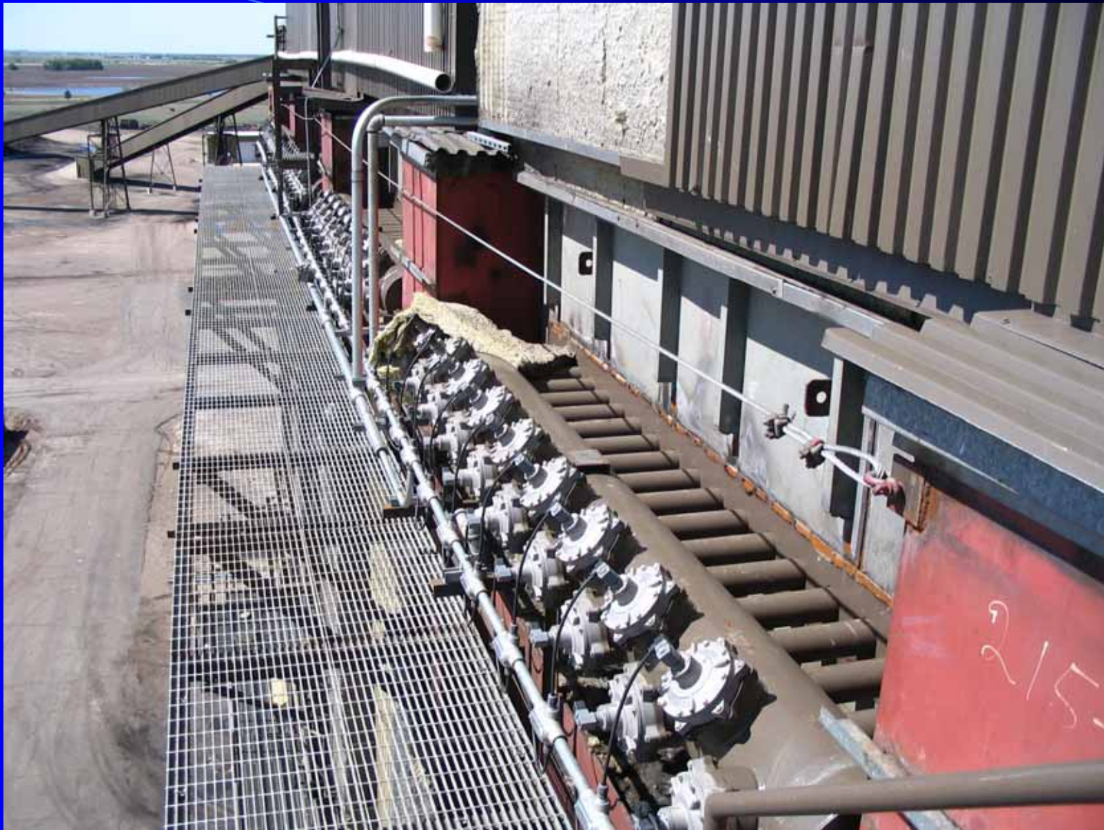
Pulse Headers – 4" Valves
