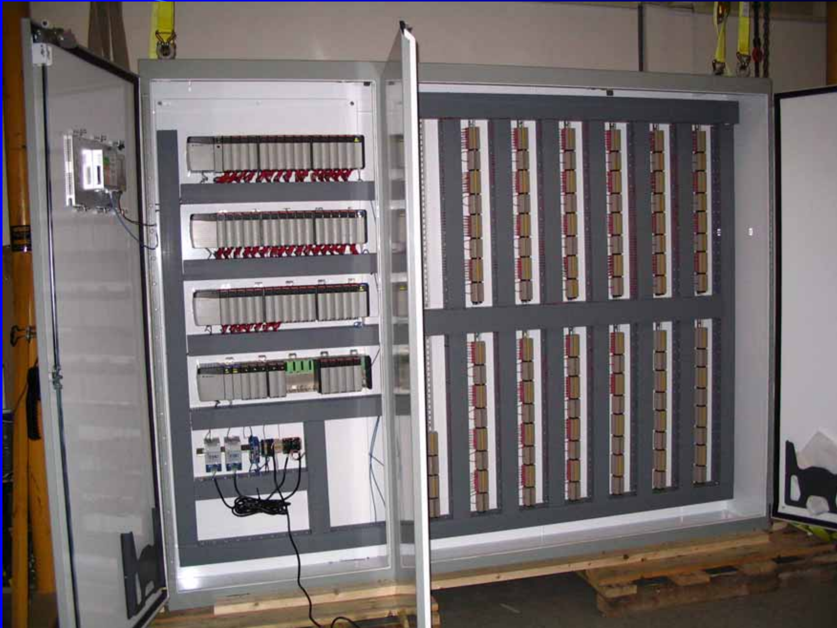
Allen Bradley Logix 500 Control Cabinet
