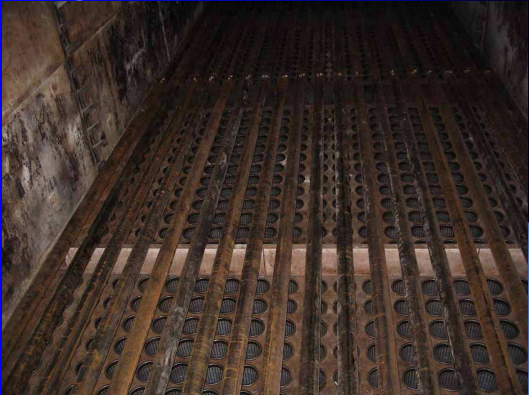
One Compartment's Tubesheet
